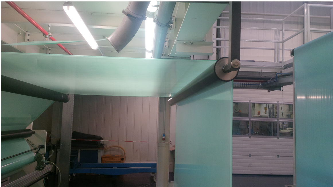
Figure 88 Polymer film process product roll main location for "cut-off" incident after extrusion and before roll-up
