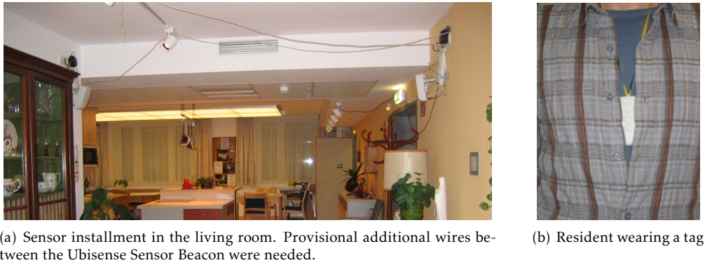
Figure 2.1: Installed UBISENSE Location System
