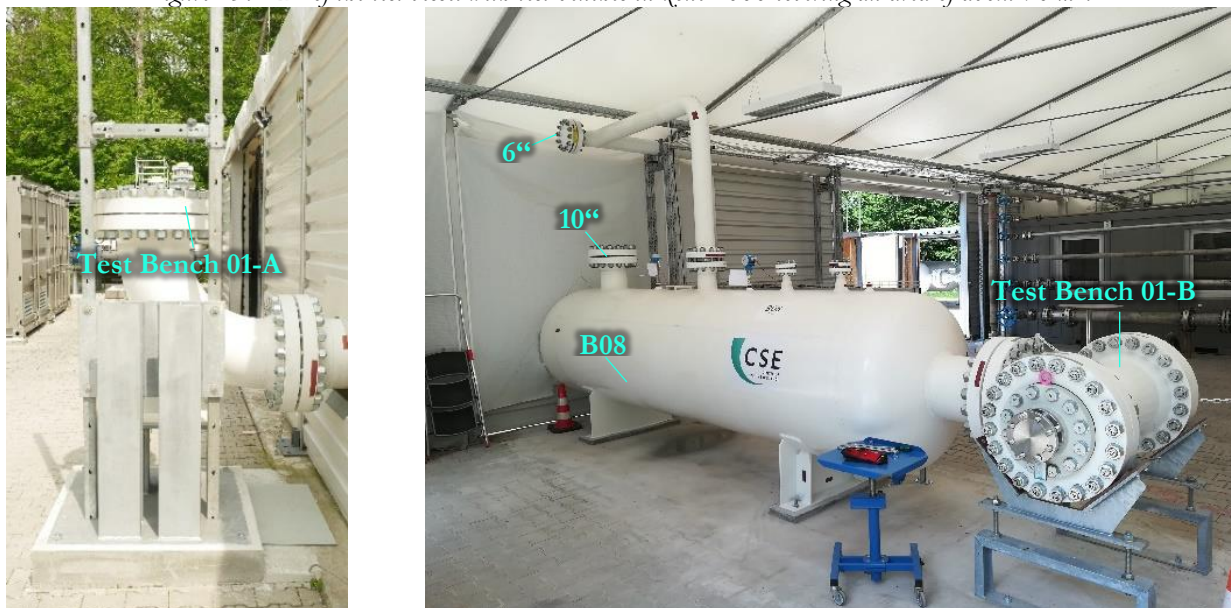
Figure 26 Images of selected components in zone 1000.
