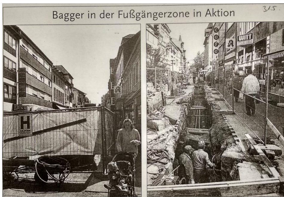
Figure 3.14. Fackelstrasse (left) and Marktstrasse (right) were under construction Source: Kaiserslautern's city archive ( Die Rheinpfalz , 31.05.1995)
