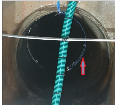
Figure 3-24 Flow measurement using NivuFlow 750 at L4 in the influent canal ( \varnothing 800 mm) of the SRT in separate system with location of the ultrasound water level sensor hanging from the ceiling and pressure unit at the lower right part of the canal
