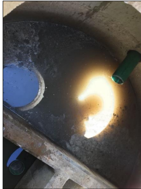
Figure 3-22 Collection and settling tank of greywater at L5.1 Reinighof on 19.19.2018
