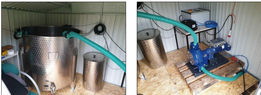
Figure 3-26 The equipment of stormwater sampling plant in separate system at L4. Left: main sampling tank and a smaller tank used for sample preparation. Right: programmable control unit, flow measurement data logger and peristaltic sampling pump
