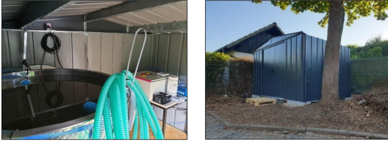
Figure 3-27 The equipment of stormwater sampling plant in combined system at L3. Left: sampling tank, surveillance camera and programmable control unit
