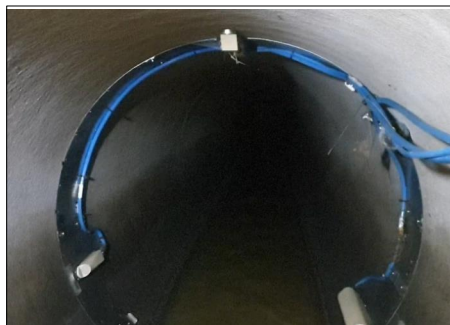
Figure 3-25 Flow measurement using NivuFlow 750 at L3 (combined sewer system) in the effluent canal ( \varnothing 800 mm) of the SRT in combined system similar to the measurement at L4. The ultrasound water level sensor hanging from the ceiling and pressure unit at the lower left side (viewer perspective). The sensor on the right is a particle quantification sensor (under development)
