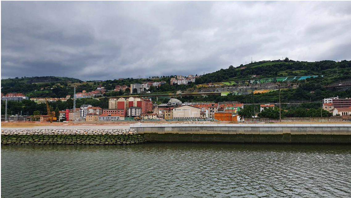
Photo 17: Land clearing activities, flood protection barriers and elevation of the level of the island are already in progress in the northern section which is inaccessible due to advanced construction works. Source: Author's archive, July 2021
