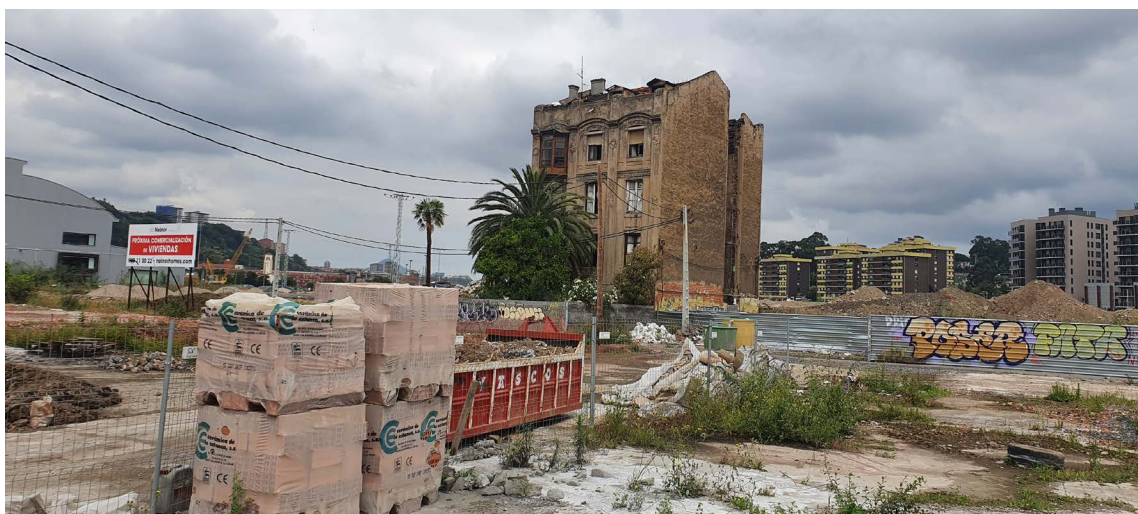
Photo 11: “La casa de la Palmera” and demolition activities in the southern part of the island and a billboard for upcoming new residential development. New residential buildings on the opposing coast to the east (the district of San Antonio) can be seen in the background. Source: Author’s archive, July 2021
