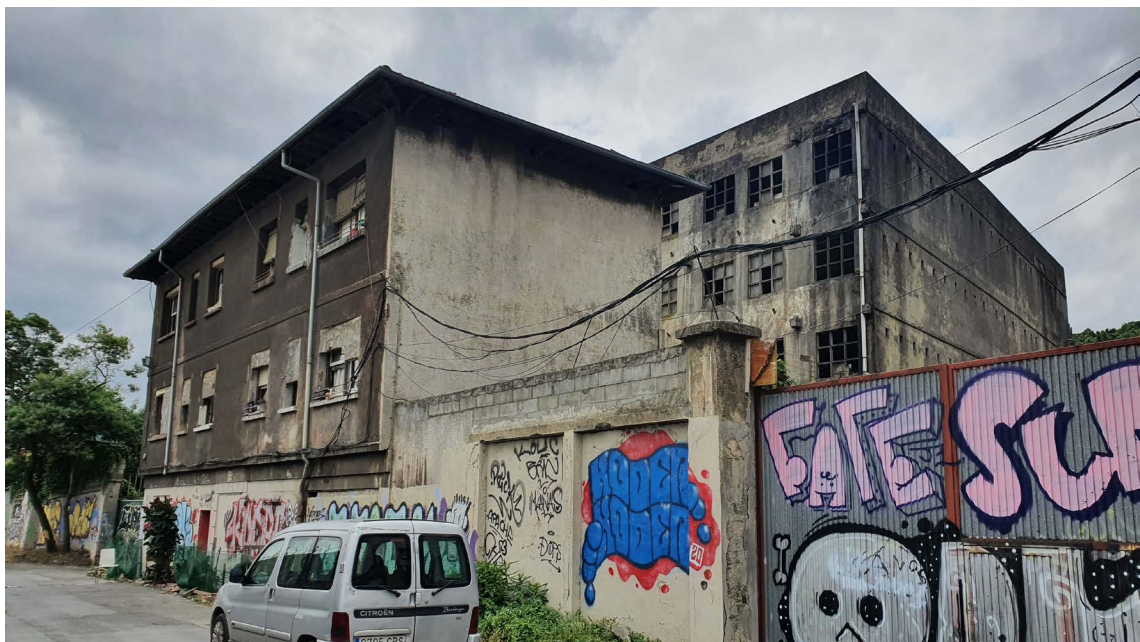
Photo 16: Residential and industrial buildings in very poor condition. The residential building appears to be illegally occupied. Source: Author's archive, July 2021
